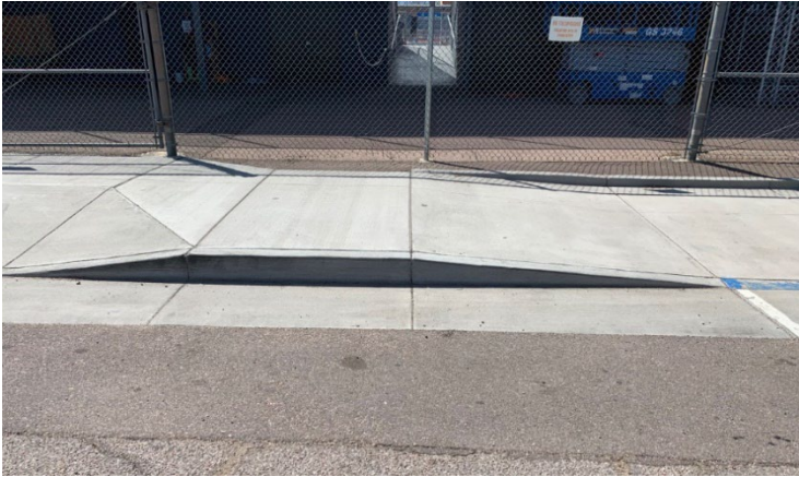
Picture 2: Site of Additional Flush Curb, Detectable Warnings (West Side of Glenn Summer Rd)
